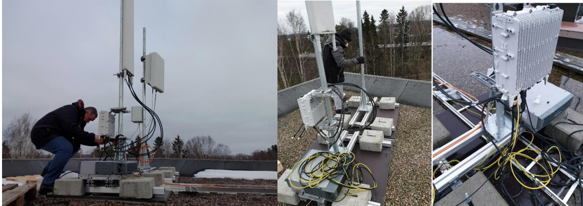
Figure 8. Aalto gNB installation in Otakaari 5 building.
